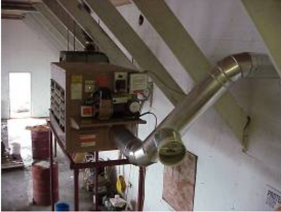
Feeding the stack from the inside of the building to the outside
