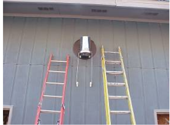
Stack coming out of the building
