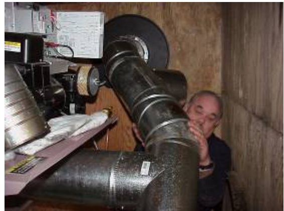
Another example of a stack being fed to the outside of the building from another used oil burner
